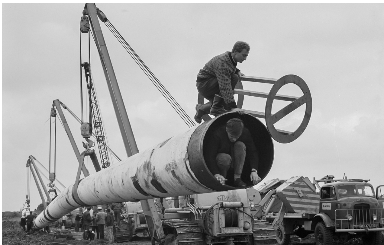
Image: The Fens gas pipeline being lifted by a row of Caterpillar 583 pipelayers. Work on laying the Fens gas pipeline started in June 1967. Over 600 men worked on the project to lay 36 inch diameter steel pipes which crossed four rivers and numerous dykes and ditches. (Heritage Image Partnership Ltd / Alamy Stock Photo)
